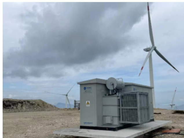
Bosnia and Herzegovina – Substation with Transformer
