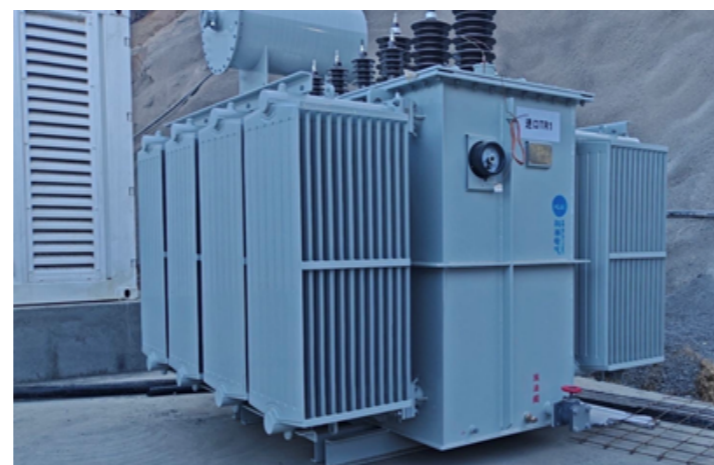
South Africa – Transformer
